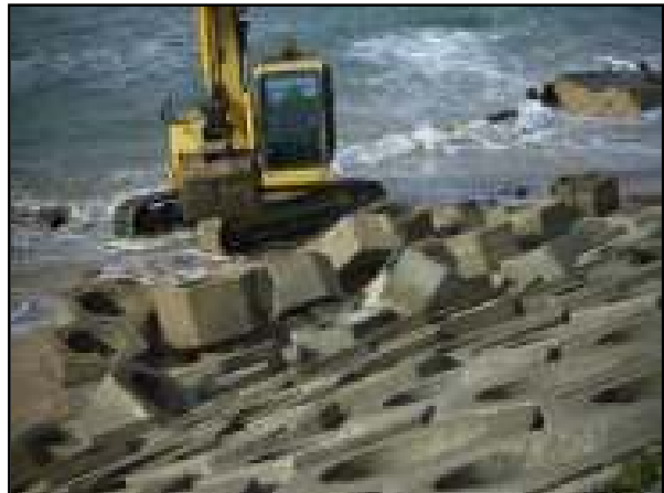
Figure 6h: Repairs to damaged seawall at Prince Street, Cronulla (Courtesy Department Environment & Climate Change)
